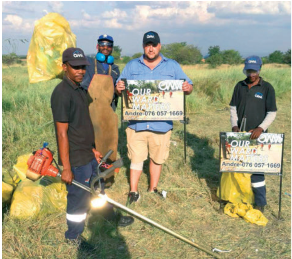
Massive clean-up efforts rolled out across Waterfall East on 26-28 March, as teams tackled illegal dumping, overgrown vegetation, and unsafe public spaces.
