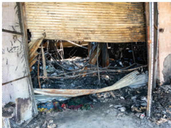
Another storage room gutted.
